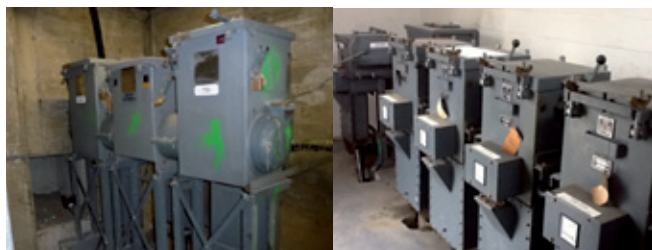
View of Long & Crawford ETV3 oil filled switch arrangement (A high percentage of these have been used in underground substations as shown above)
